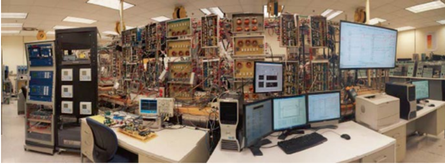
Fig. 3.6 A view of the Smart Grid testbed at Florida International University (FIU)
